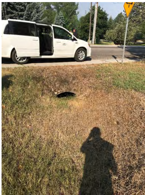
Figure 4.3.6-1 Plugged culvert between Jack Dr. and Helena Dr.
