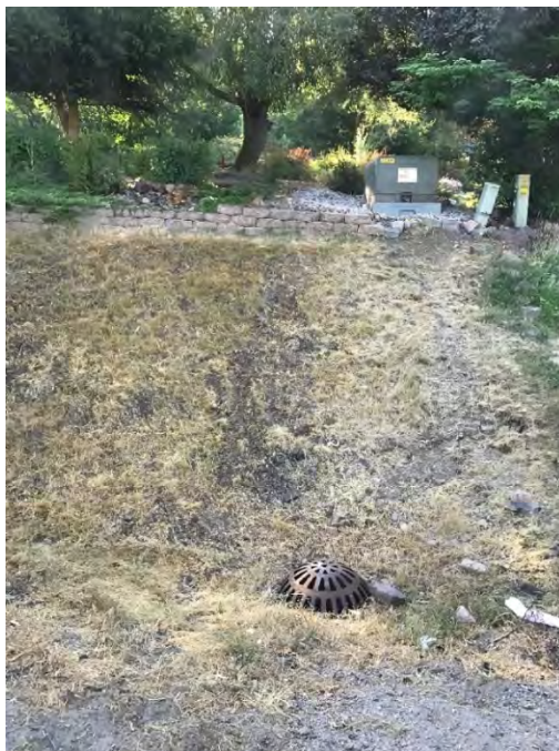
Figure 4.3.2-2 Drainage ditch with beehive grate inlet
